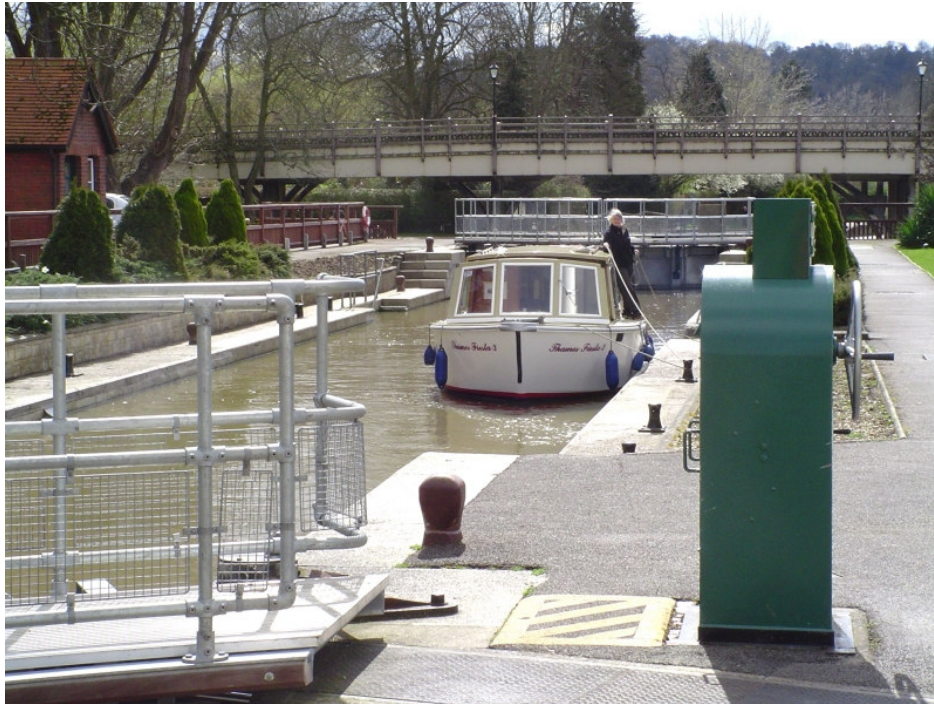
Goring Lock, River Thames – Photo shows user operated control station with both manual and computer sequenced operations.
