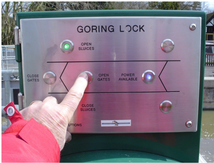
Boat crew's operating panel at Goring Lock
